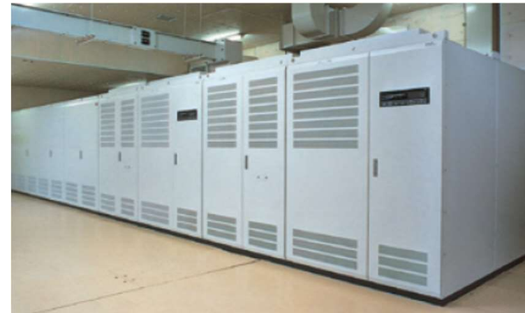
Internet data center (IDC)
